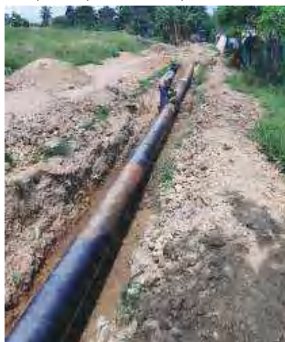
Pipeline system for transportation Fuel
