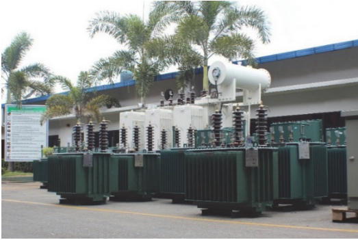
Transformer Plant at Angulana
