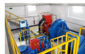
Turbine and Generator
