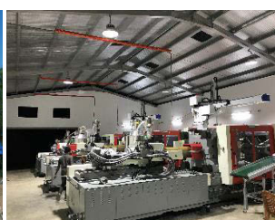
3 Injection Machine Unit
