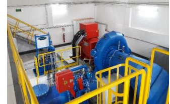
Turbine and Generator
