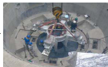
Braodlands Power House
